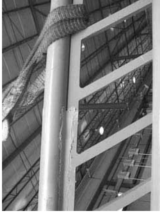
Lab-metal is applied with a putty knife to finish a rough weld. The hardened Lab-metal is then sanded smooth, providing a paintable, permanent metal finish.
