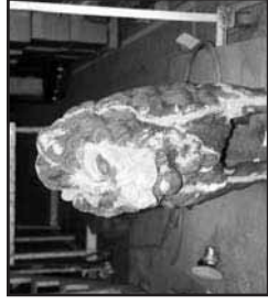
Before and After: Hi-Temp Lab-metal was used to patch cast iron lion statues in an historic restoration project.
